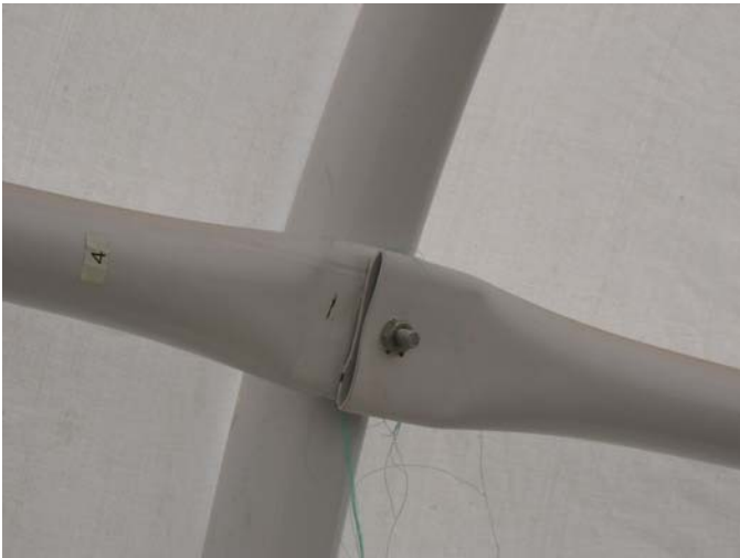
Cross Rails inside Frame Overlapped on Same Bolt
